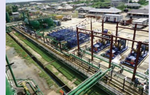
Aerial View of Liquid Treatment Facility
