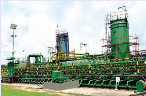
Oben Flow Station
