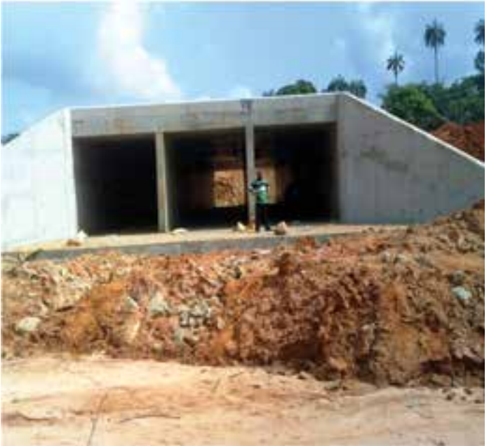
Erosion Challenge in Auchi (After intervention)
