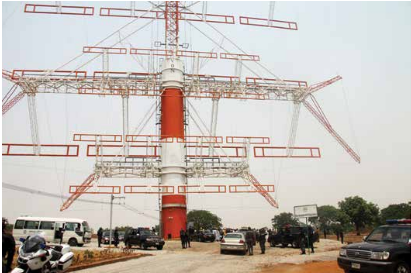
Multi-billion Naira Revolving Transmitter of the Voice of Nigeria in Lugbe, Abuja
