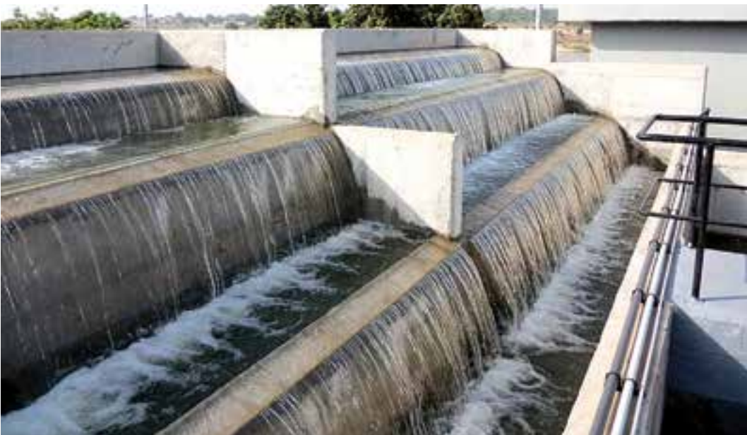
The Otobi-Otukpo Water Works, Benue
